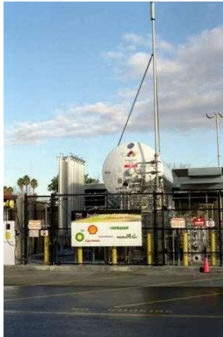
Figure 16. Cryogenic liquid hydrogen storage tank.
